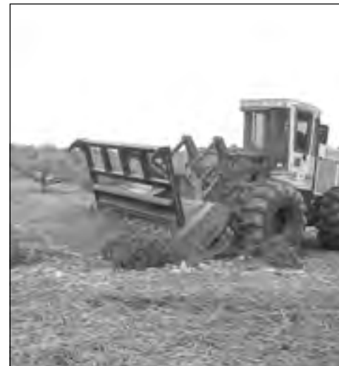
A piece of Cedar Eater heavy equipment clears land. The company uses specialized tools for cutting down cedar, mesquite and other trees.
